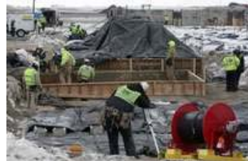
John M. Steiner / The Sun Construction workers brave the elements Tuesday in Spiritwood as they work at putting in footings on the frozen site of the future Great River Energy power plant.
