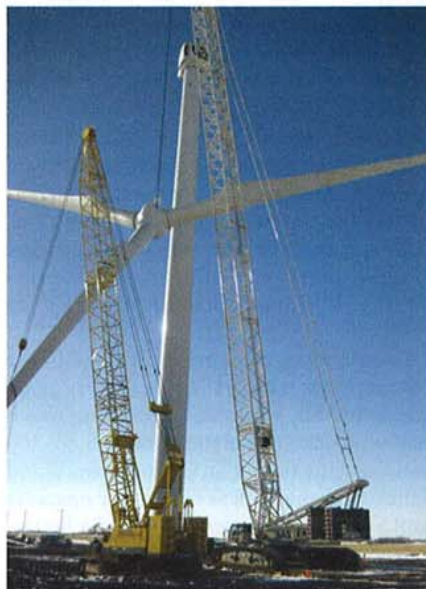
Wanzek Construction's Demag CC-2500-1 (550-ton) and Kobelco CK1000 (100-ton) installing rotor on wind tower at the Endeavor Wind Farm near Harris, Iowa
